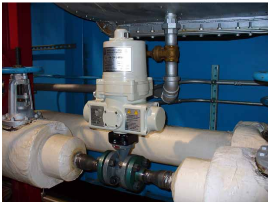
PA Spring Return Actuator, 24 vac, controlling condensate in a chiller system. This model has no manual handwheel.
