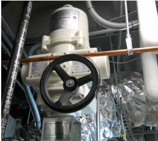
PAO Spring Return Actuator on a damper for air handling.
