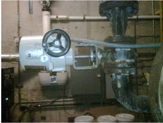
A P5-120-N4 Actuator with Torque Switches on a Cooling Tower Control Valve
