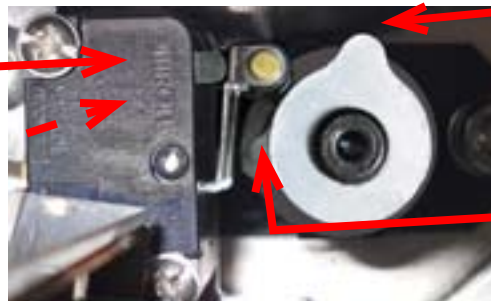
Torque Switch cams shown in the NORMAL operating position (No high torque situations)
