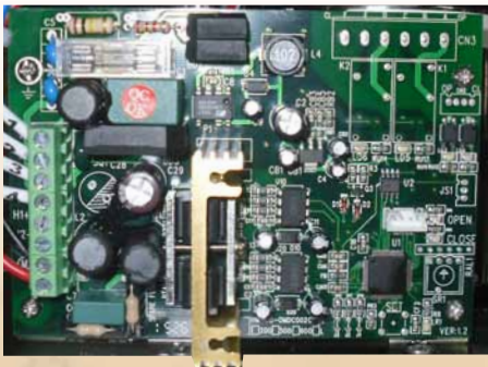
Control Board supplies power and control to the 125vdc motor.
